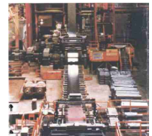
Bandverzinkungsanlage Belt-type galvanizing plant
